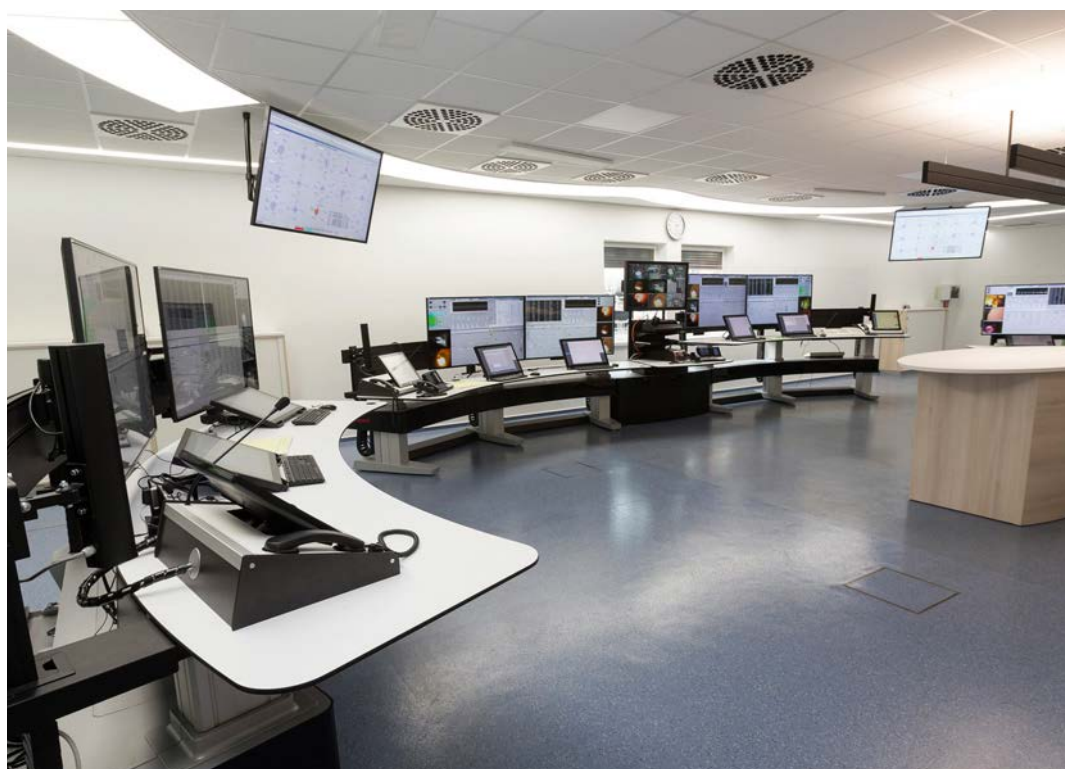
Measuring station for residue incineration at BASF Ludwigshafen
